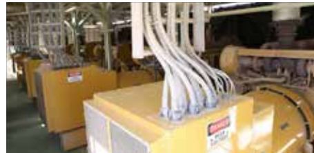
Fig 9.5 – Rig power engines
