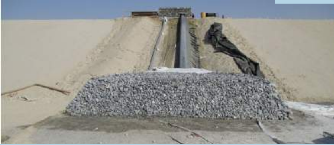
Figure 5.16 North-Kuwait Landfill- Leachate Collection Riser Pipes
