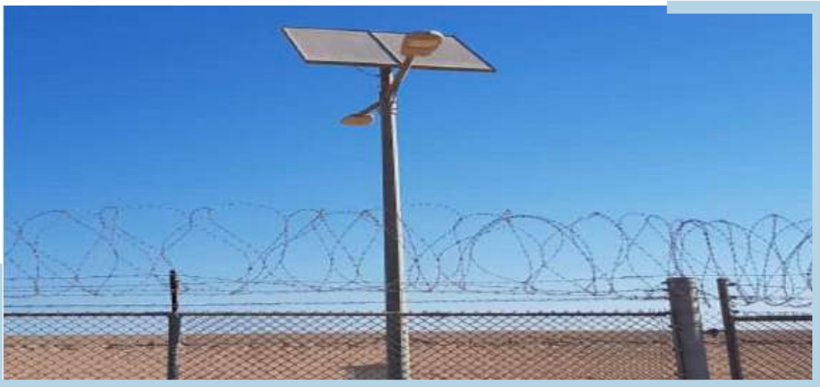
Figure 5.23 South East-Kuwait Landfill- Solar Panel and Light Pole
