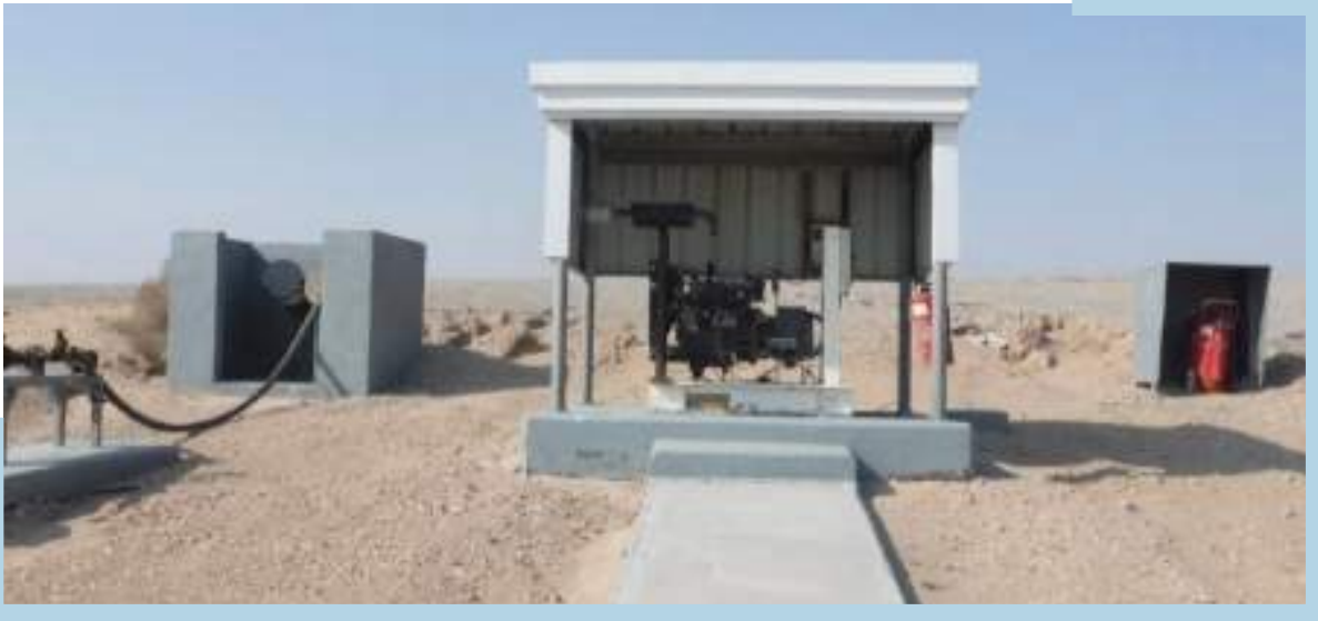
Figure 5.22 South East-Kuwait Landfill- Leachate Riser Pipe and Generator
