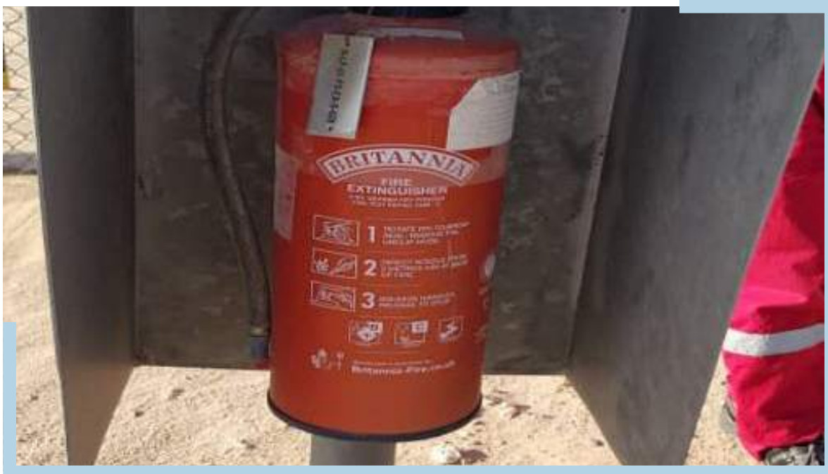
Figure 5.24 NK Landfill Fire extinguishers
