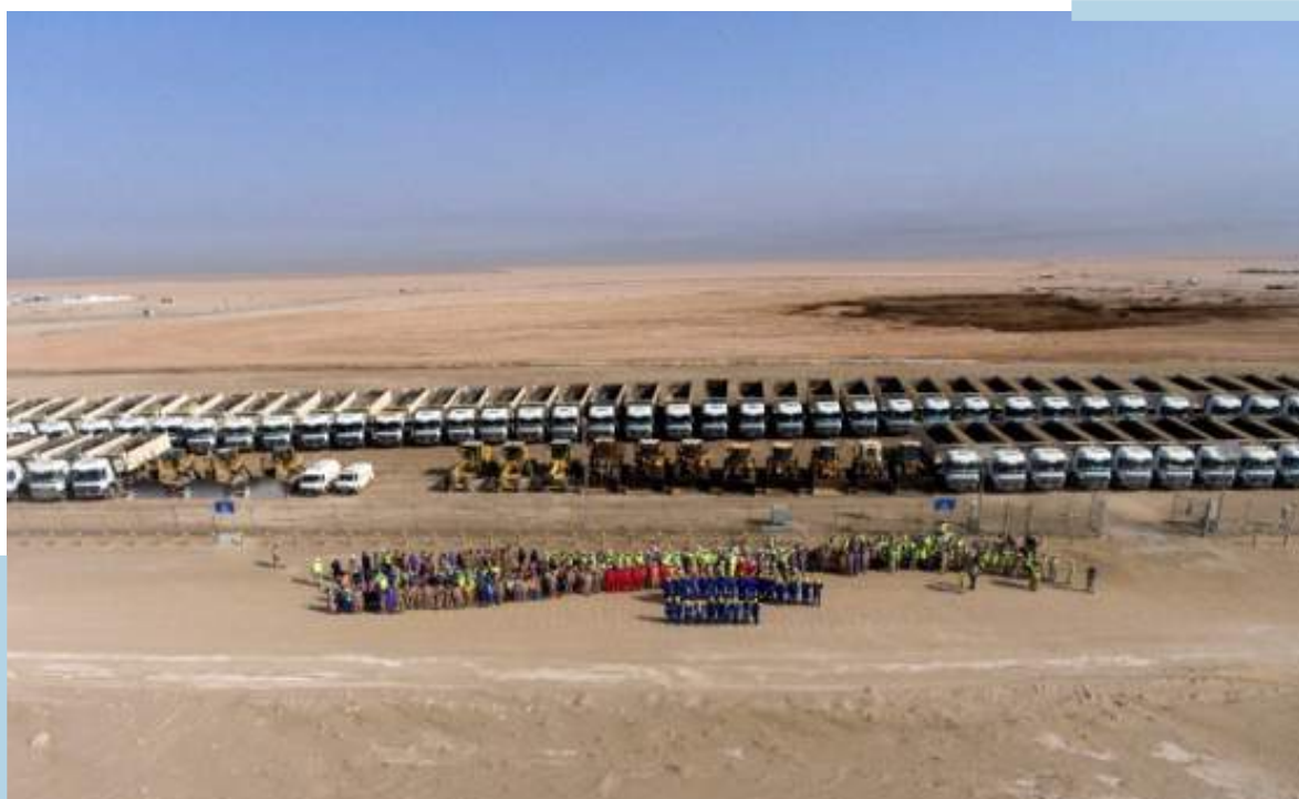
Figure 5.52 Final Day & Celebration of the NKE&T & Infilling of the landfill with Oil Contaminated Soils
