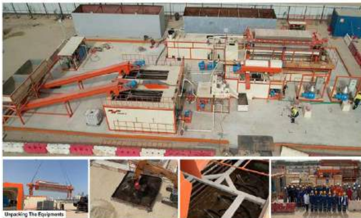
Figure 6.42 Field Trials works for portion 4 utilizing Soil Washing Treatment for SKETR Zone 2
