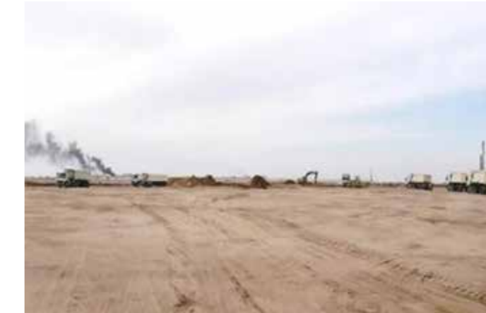
Figure 27. Dry oil lake after remediation by KOC.
