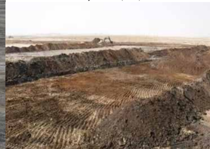
Figure 26. Dry oil lake contaminated area before remediation.
