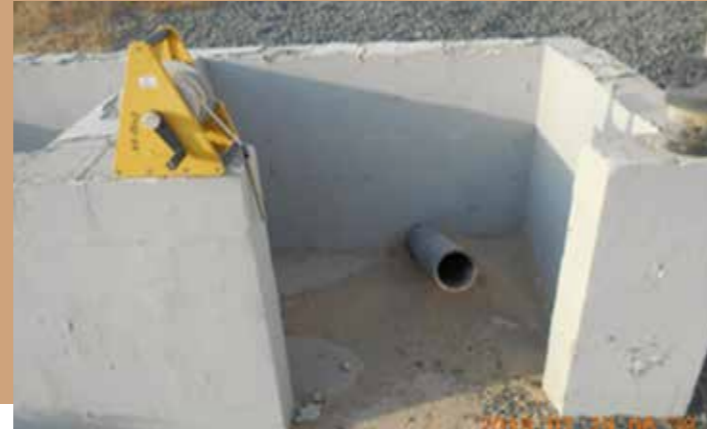
Figure 38. Leachate Inspection Pipe in the landfill.
