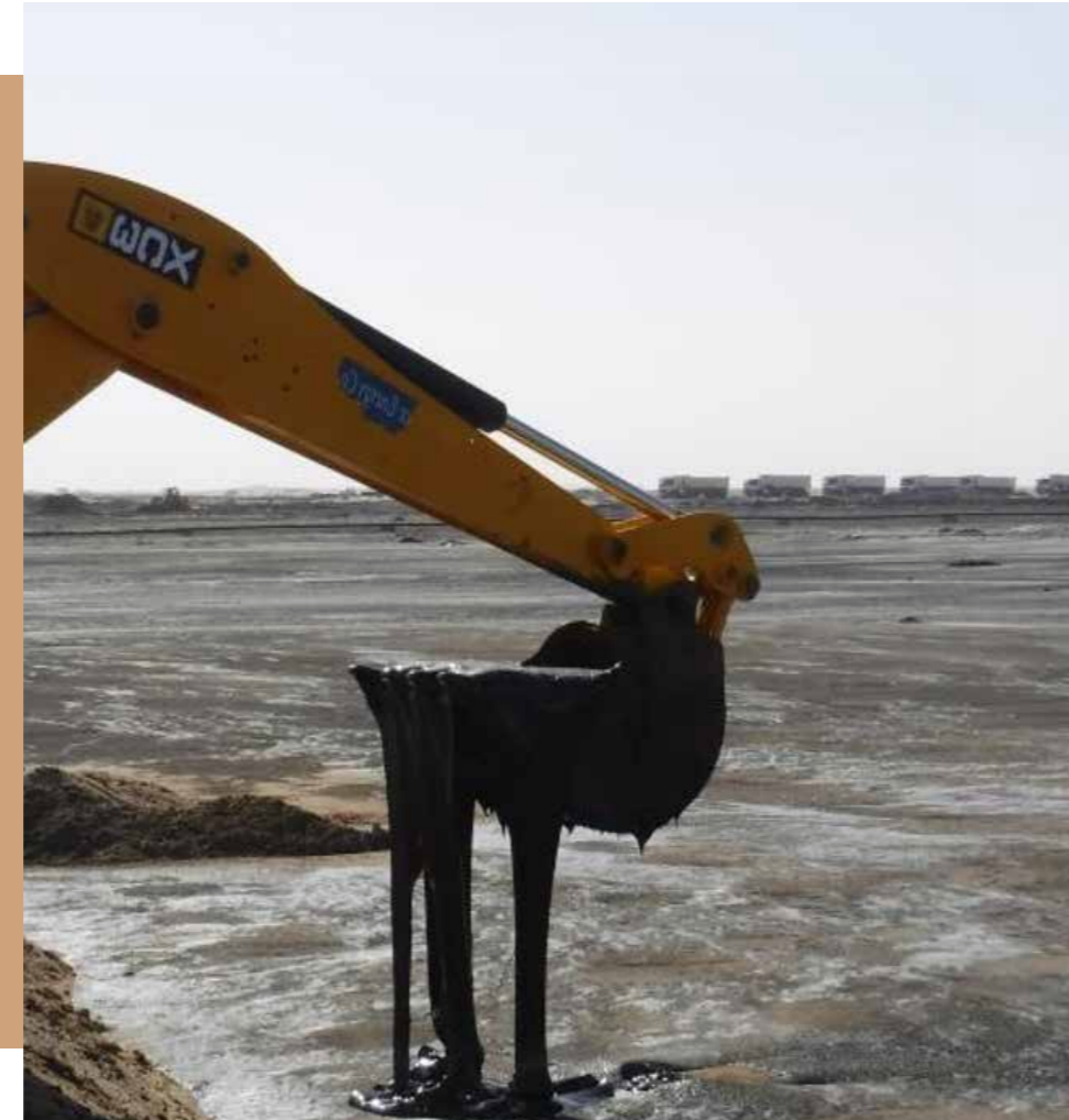
Figure 24. Wet oil lake before remediation (2016)
