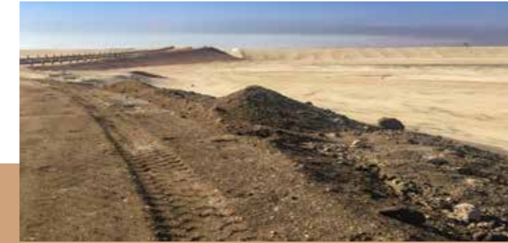
Figure 14. Early stages of landfill construction and filling in the North area of Kuwait (S)
